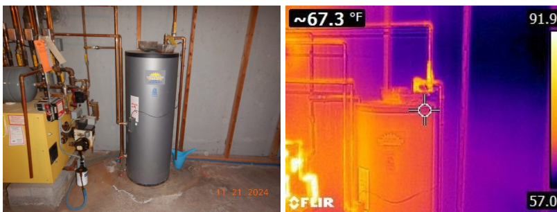
IR Hot Water Heat Tracing
