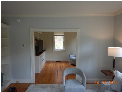
Racked Door Frame As A Result Of Floor Deflection
