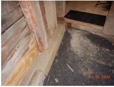
Twisted Lap Sill Repair
