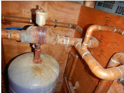
Leaking And Corroded High Air Vent
