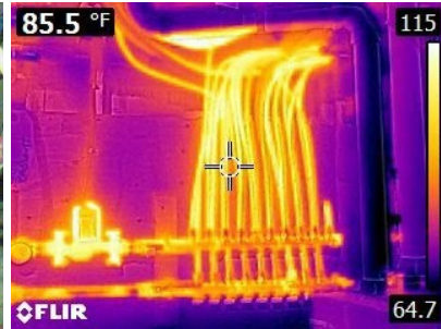
IR Upper Floors Radiant Floor Heat Tracing
