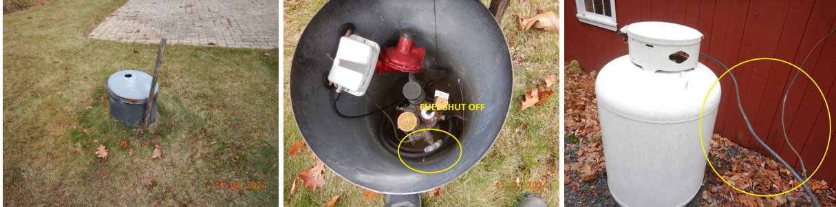
Improperly Secured Full Line
